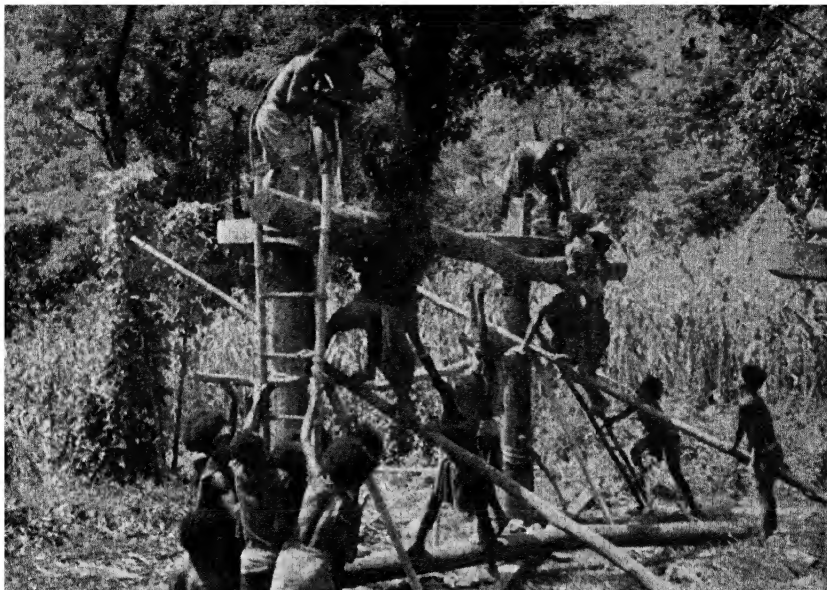
Placing a floor beam on the house posts. Note the rat disks like wooden collars on the house posts.
